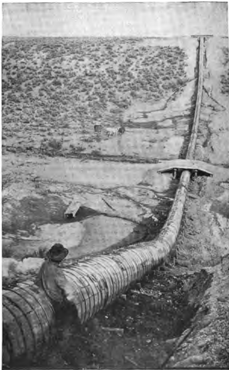
FIG. 148.—Continuous Wood-Stave Pressure Pipe, Idaho Irrigation Company's Canal.
